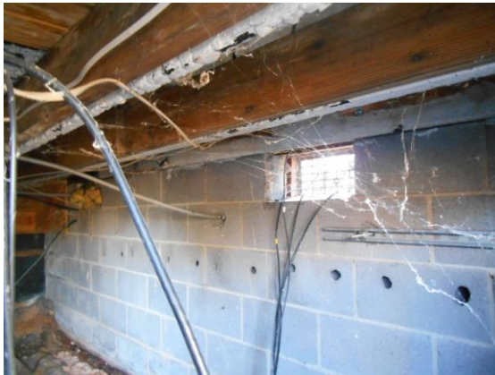
Coax Entering Building
