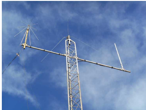
Reidsville Red Cross Antenna Tower
