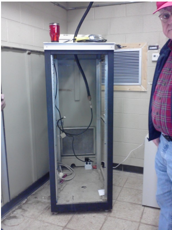
Illustration 1: Gutted Empty Equipment Enclosure
